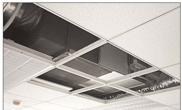
Lossnay installed in attic.
