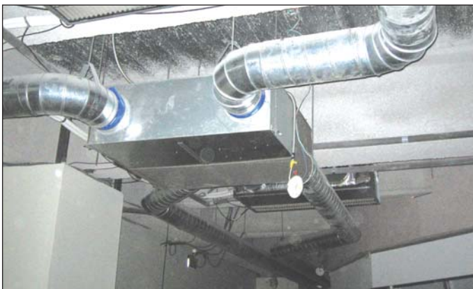
Lossnay installed in attic.
