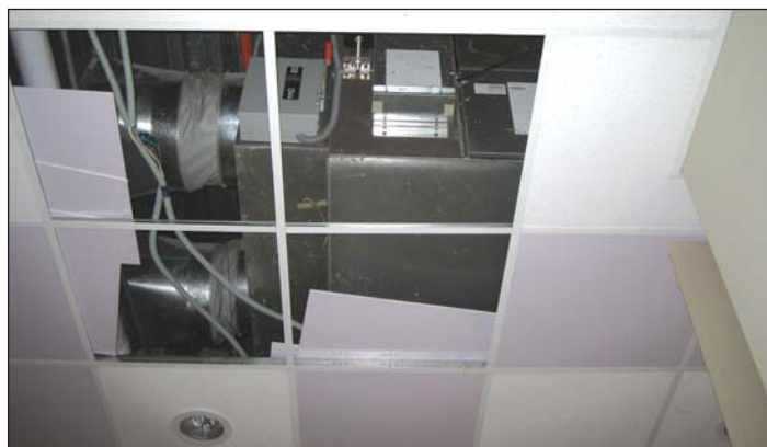
Lossnay installed in attic.
