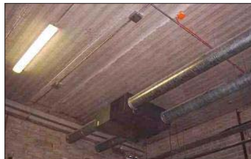
Lossnay unit is suspended from ceiling.
